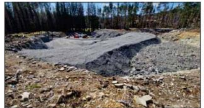
PARKED UP: Works vehicles in the borrow pit gives an indication of the size of the excavations that have taken place on Balavil Estate.
